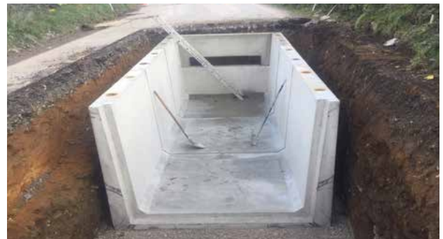
Figure 11: A typical jointing bay where cables are connected
