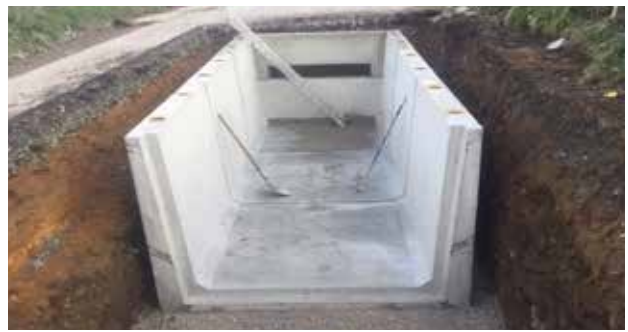
Figure 12: A typical jointing bay where cables are connected
